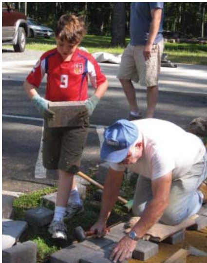
Nathan Jordan assists Don Willock in laying the front patio leading to the Lighthouse.
